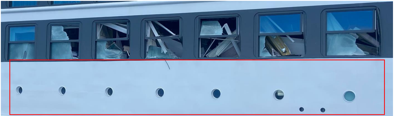
Figure 14-1 Undamaged steel. The maximum pressure these plates can withstand has been calculated in Stipla.
