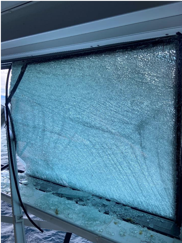
Figure 26: Broken window in stateroom 2016. Photo: NSIA
