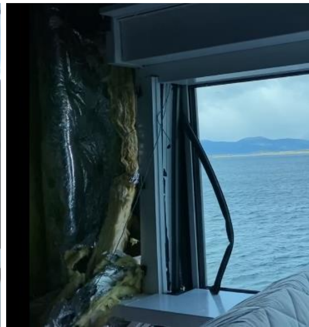
Figure 31: Damage to upper window frame in stateroom 2020. Photo: NSIA
