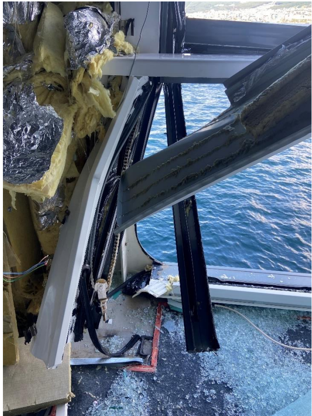
Figure 25: Damaged window frame in stateroom 2014. Photo: NSIA
