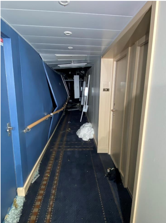
Figure 36: Damage to corridor viewed from staterooms 2010 and 2012 on deck 2, view towards the stern. Photo: NSIA
