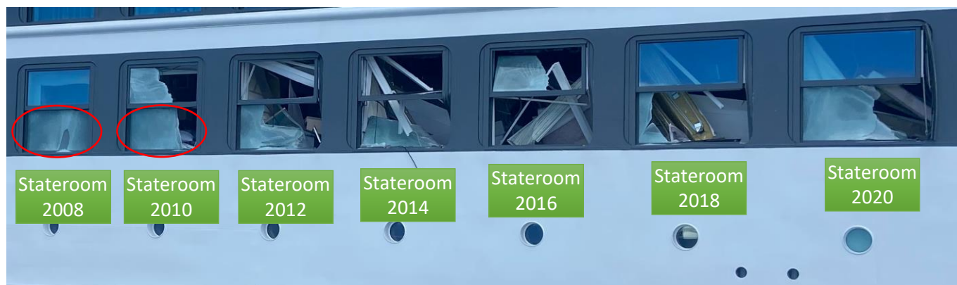
Figure 9-9 Overview photo showing the damaged staterooms on deck 2.
