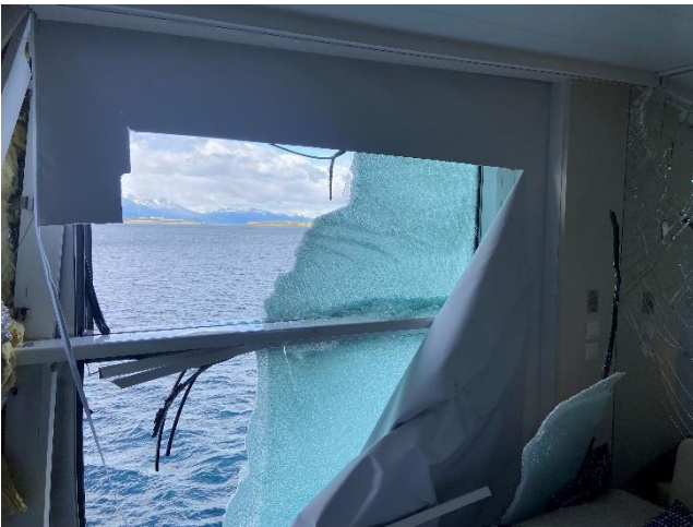
Figure 21: Damage to window and frame in stateroom 2010. Photo: NSIA
