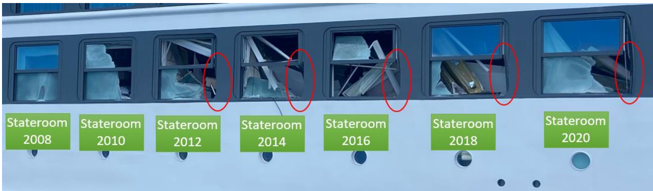
Figure 74: The overview photo shows the damaged staterooms on deck 2. The staterooms where the aft frame post was knocked in on five of the seven damaged windows are circled in red. Photo: NSIA/consultant
