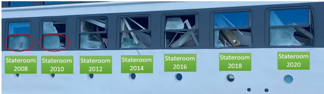
Figure 76: The windows where the window pane is broken but the frame is intact are circled in red. Photo: NSIA/consultant
